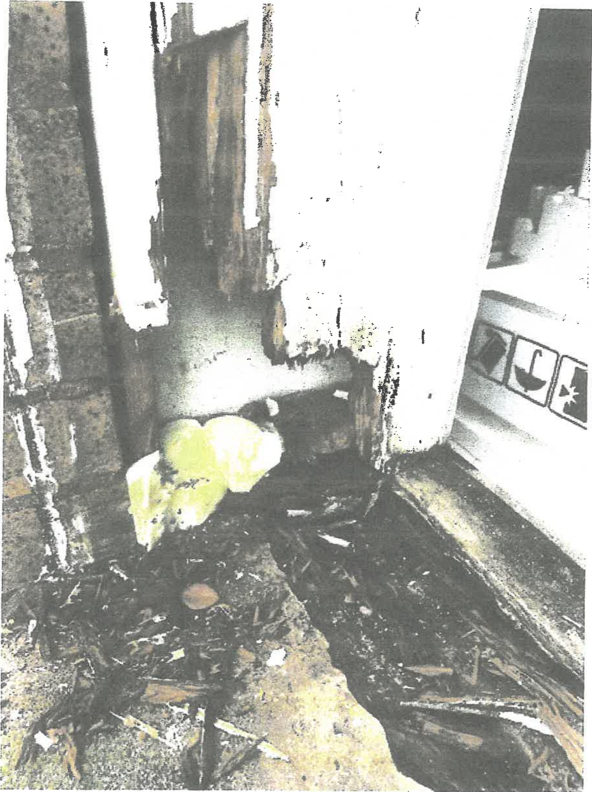
Chase Bowen Rotted Window removed
