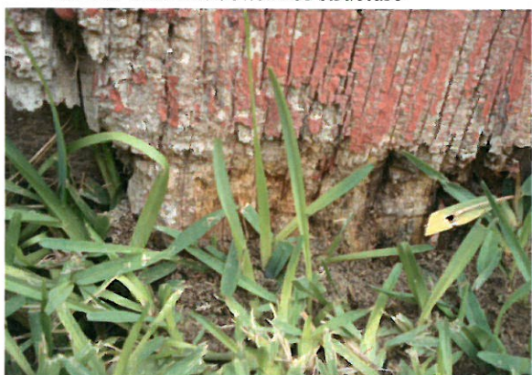
Siding is rotted up several inches from ground
