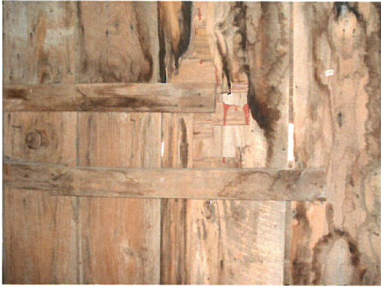
Interior Rotted Wood and Water Damage
