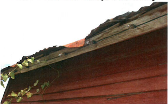
Sheet Metal is not secured to roof
