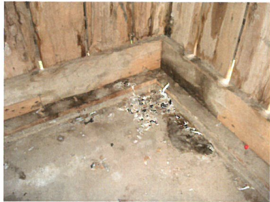
Water penetrates through roof and floor
