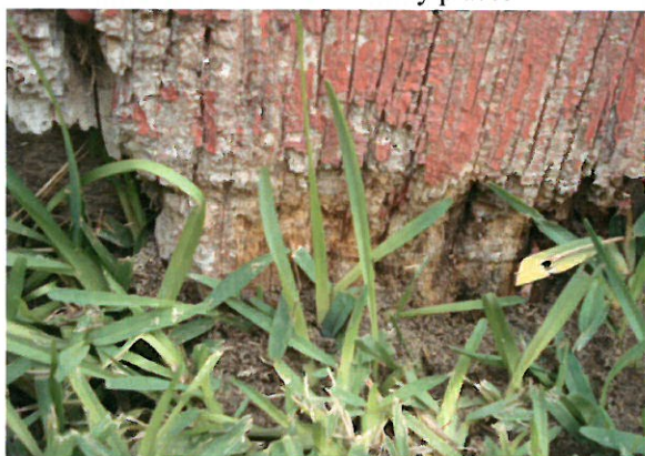
Structure is very unstable in its current condition
