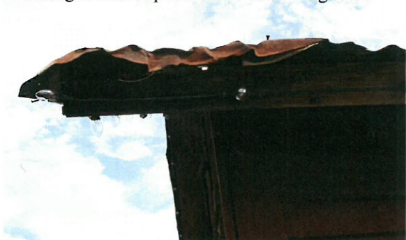
Damaged Siding is a Safety issue if high winds
