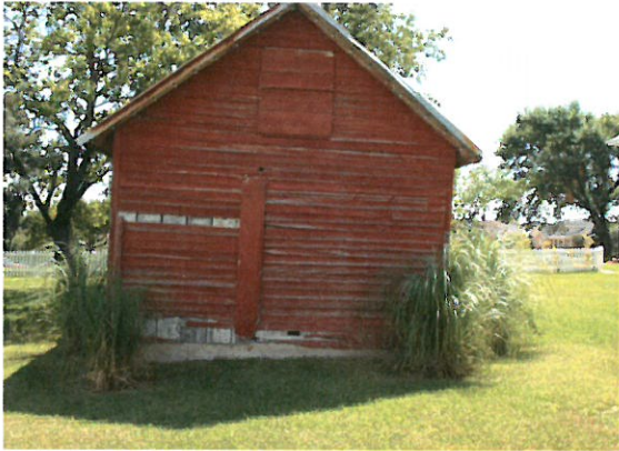
Photo of Barn leaning over
