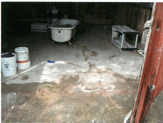
Water seeps in during rain
