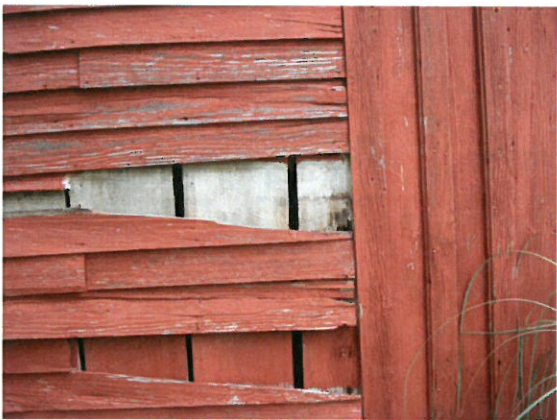
Missing Siding in many locations/Gaps
