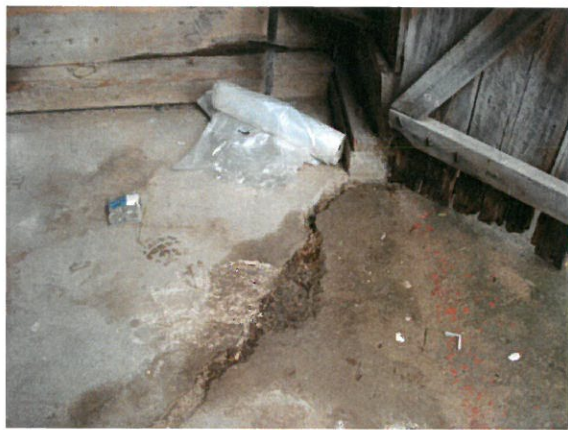
Foundation is cracked in many places
