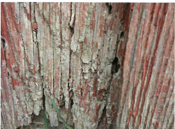
Rotted wood/Termite Damage/Water Damage
