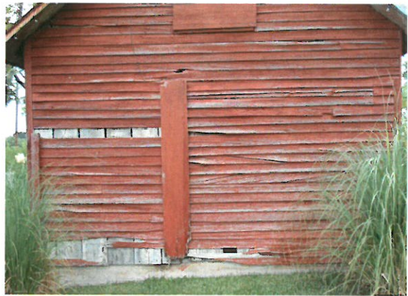
Rotted and Missing Siding
