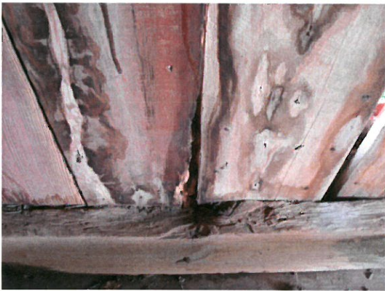
Water penetration prevents use as storage
