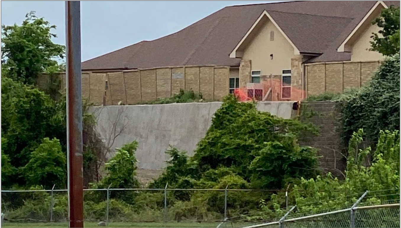
FIGURE 3. PICTURE SHOWING THE EXISTING SPLIT FACE CMU BLOCK WALL AND THE NEW SMOOTH FACE CONCRETE WALL.
