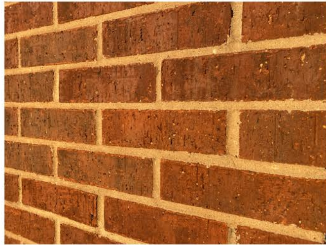
A BRICK VENEER: FIELD COLOR TO MATCH EXISTING BUILDING ACME, COLOR - QUORUM
