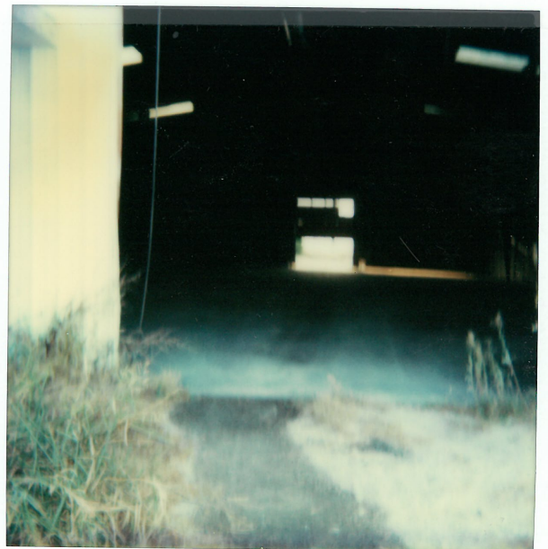
Present appearance of shop interior, (note overhead doors badly decayed.) Doors are to be replaced
