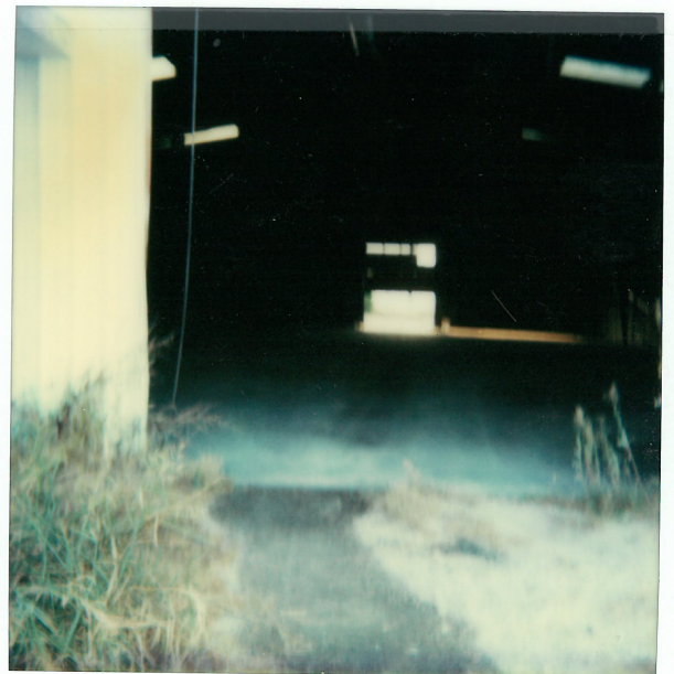
Present appearance of shop interior, (note overhead doors badly decayed.) Doors are to be replaced
